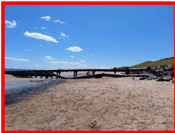
Failed and disused outfall – H&S risk (/3901C05)
