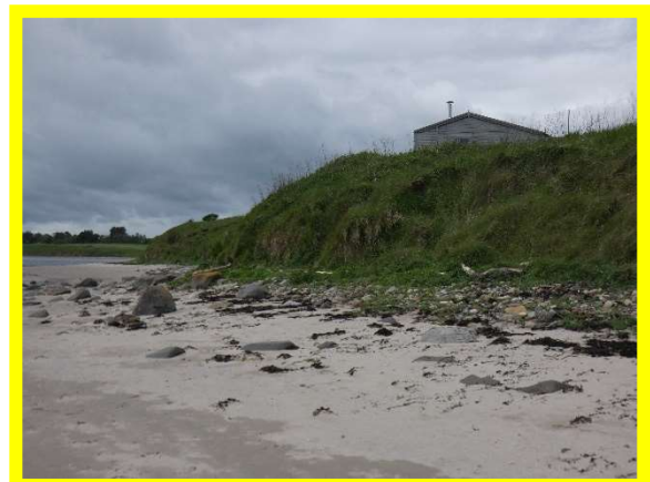
2601/C07 on-going erosion to cliff south of Seaton Point.
