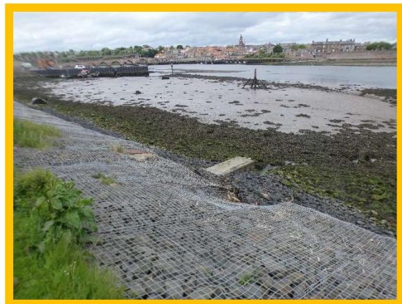
901c04 continued damage 2022.
