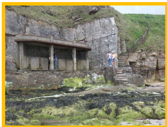
Concrete pavilion structure in fair/poor condition, missing brickwork from fronting wall (/0701C02)
