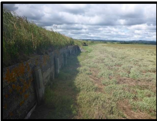
1401C98 – (Photo from 2020) retaining structure in fair condition. Rotten timber support posts and minor rotational movement.
