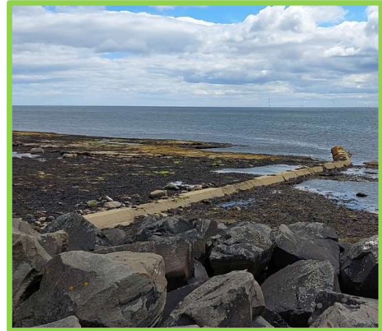
Outfall crossing underneath the North breakwater in Newbiggin Bay in overall good condition (/3601C14)
