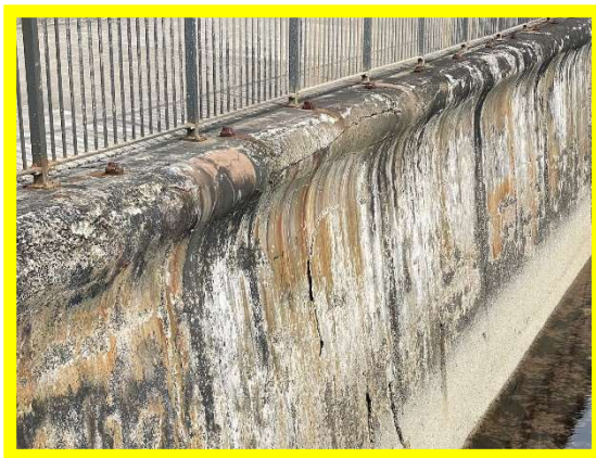
Seawall in fair condition with corrosion, spalling and some cracking, this is typically limited to the cope (/3101C05)
