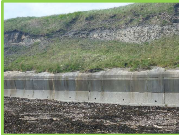
Sea wall with slumping cliffs above (/4401C18)
