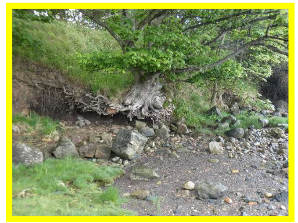
1501/C05 – local bank failure but no apparent risk to road.
