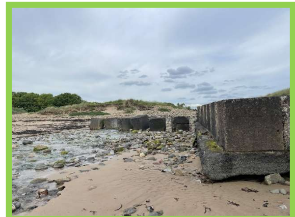
Drainage occurring alongside of remnant outfall structure through gravel, cobbles and boulders (/3201C09)
