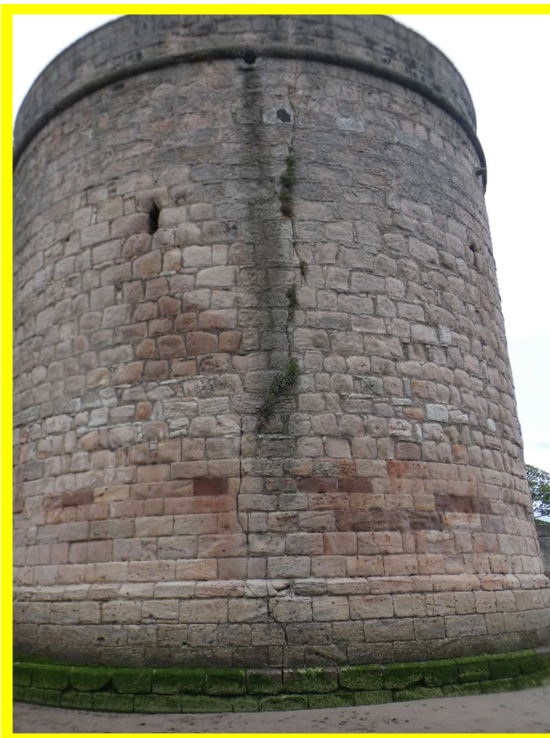
Vertical crack in wall at roundhead (/0801C06)
