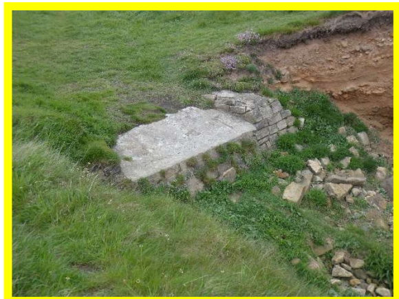
2401/C02 outflanking of local masonry wall to south of Rumbling Kern. No worse than 2020.
