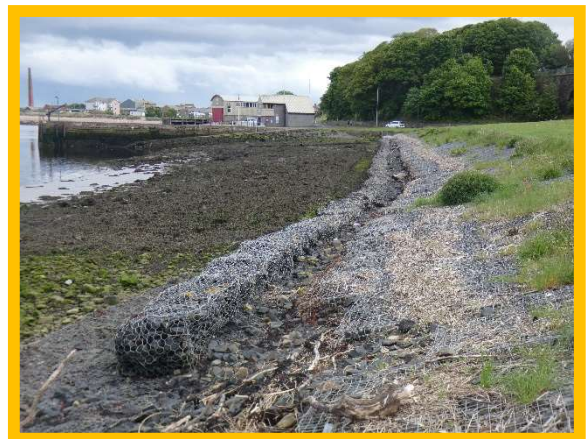
901c04 continued damage 2022.
