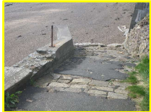
Abraded access ramp (/4401C16)
