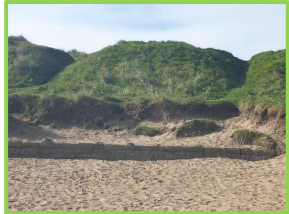
Southern wall in fair condition with some dune erosion behind (/4301C02)
