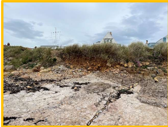
Ongoing erosion to slopes fronting properties (1701C44)
