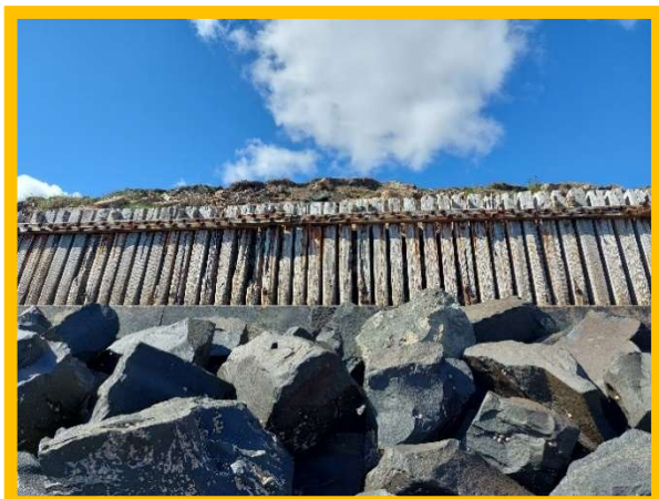
Corroded holdings and rotten timber screen – are in poor conditions and requires repairs (/4001C03)
