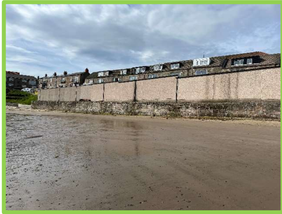
Good condition overall – areas of fair condition where cope is breaking away with vegetation growing through (1701C15)
