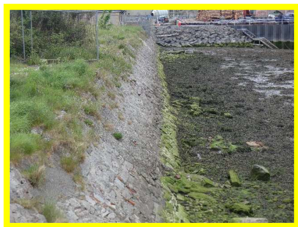
Minor loss of pointing 2020
