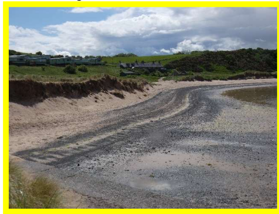
1501/C06 – continued erosion of dune 2022
