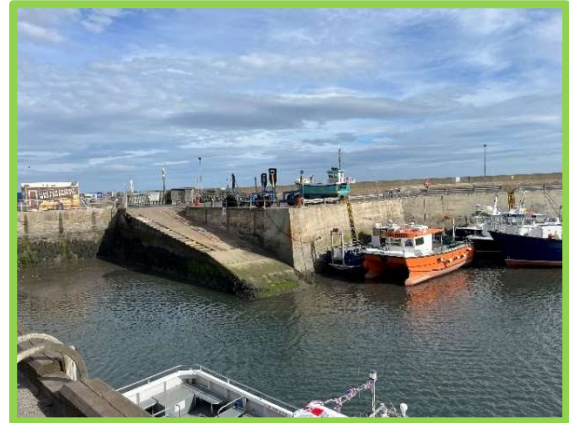
Undercutting of slipway not visible 1701C12
