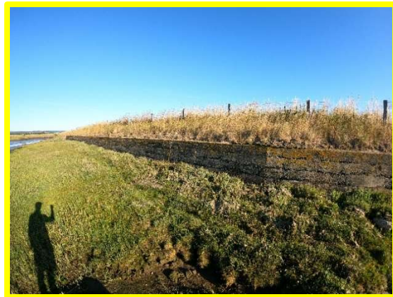
1401C13 – Heavily abraded concrete retaining wall
