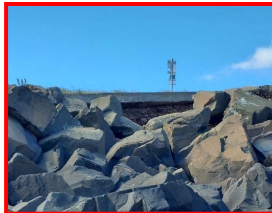
Ramp concrete slab undermining – needs to be repaired (/4001CO1)
