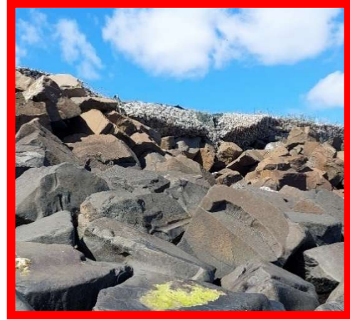
Localised cliff slide producing revetment movement and gabions failure on top of cliff (/4001C01)
