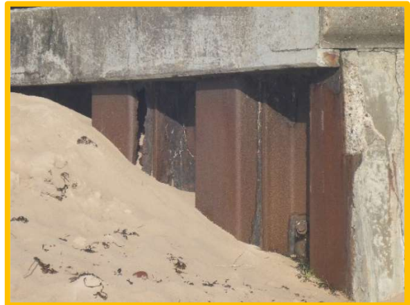
Voids in steel sheet pile end to promenade (/4201C08)
