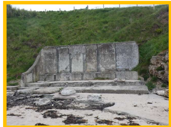
Short seawall with active breaking-up apron (/0701C07) 2022
