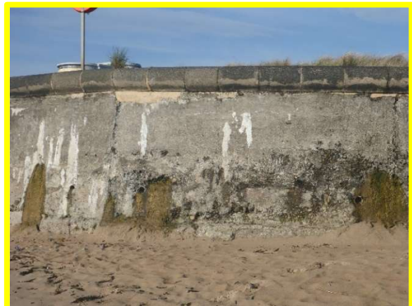
Abrasion and staining to sea wall at its northern end (/4201C06)
