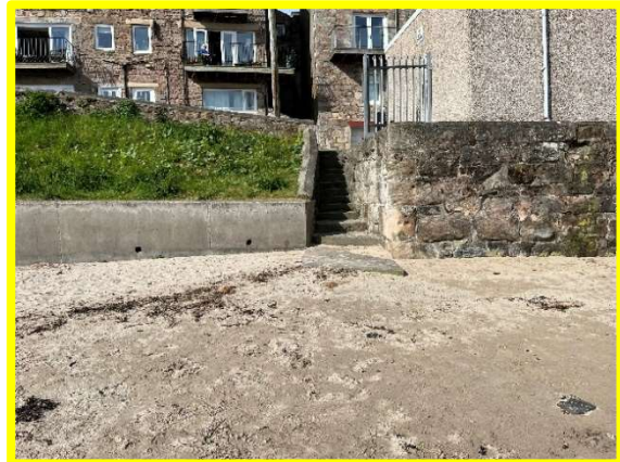
Undercutting of toe of steps concealed (1701C16)
