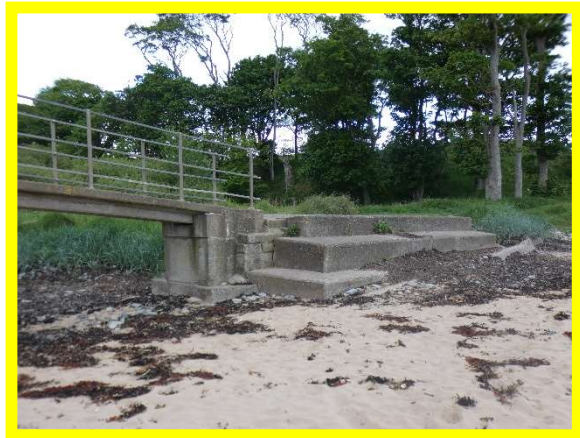
2501/C01 lower beach levels around supports to northern side..
