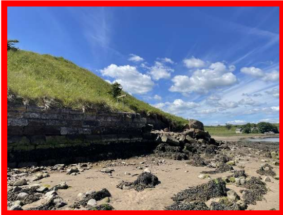
Collapsed section of wall at Church Hill with erosion of the land behind (/2801C13)
