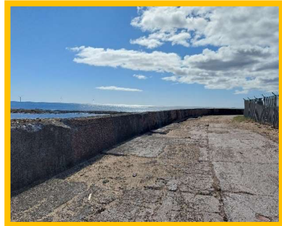
Parapet in poor condition with missing and broken walkway slab sections – signs of undermining (/4001C04)
