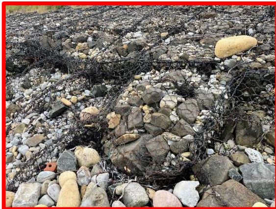
Failed mattresses at Beadnell North (Lady's Hole) (1701C39)
