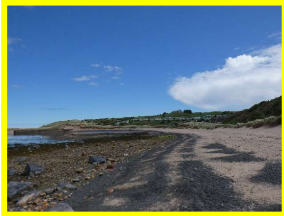
1501/C06 – erosion down to stone on foreshore south of Jetty
