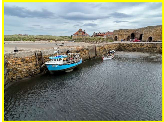
Missing blocks at Beadnell Harbour wall (inner face of northern wall) (/1701C52)
