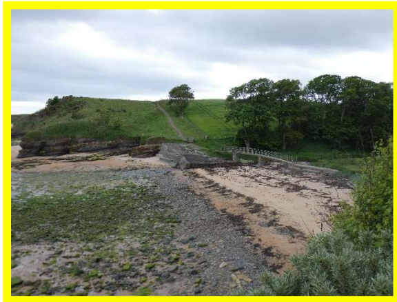
2501/C01 Undermining of concrete at southern bridge abutment. However limited deterioration since 2020.
