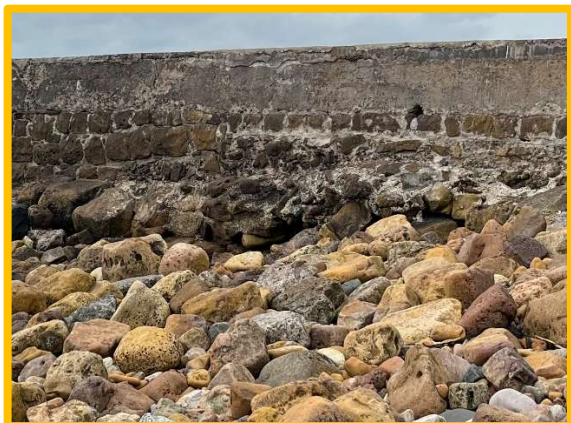
Potential voiding beneath outer face of pier adjacent to rock armour (1701C47)
