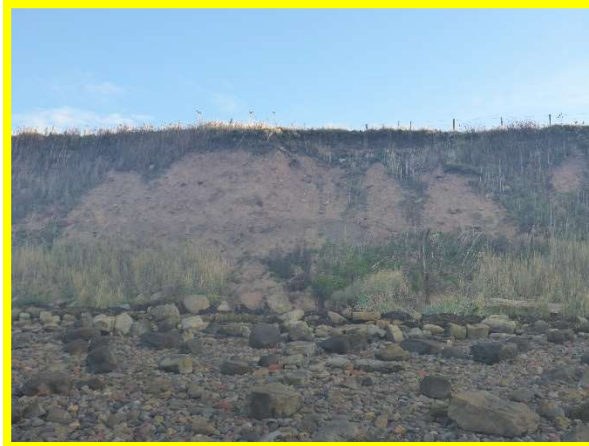
Eroding section of higher cliff (/4901c03).
