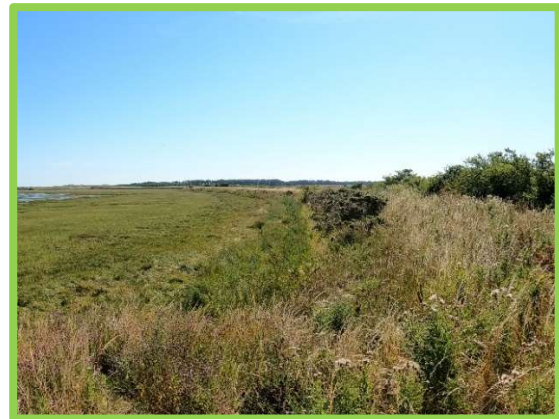
1401C98 – Densely vegetated embankment.
