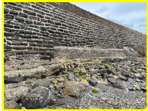
Repaired section of abraded concrete toe at Beadnell North (Nacker's Hole) (1701C36)
