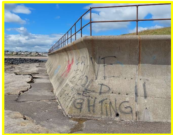
Recurved section of Church Point seawall in good condition. Toe apron cracked. Rusty handrailing (/3601C13)
