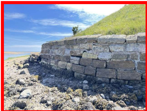
Displaced blockwork in wall at Church Hill (/2801C13)
