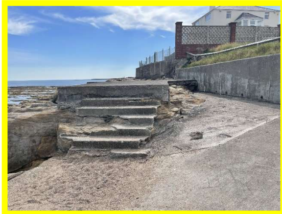
Heavily abraded access steps to Pan Point (/3101C02)
