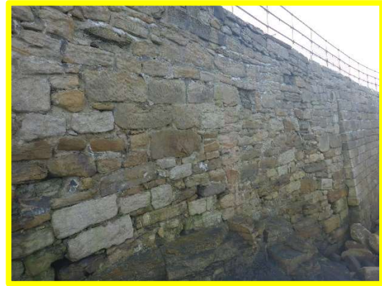
High masonry wall (/4401C11)
