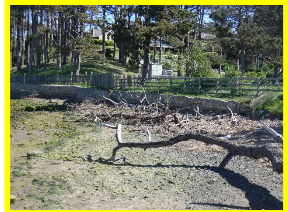
2801/C10, slight damage to downstream end.
