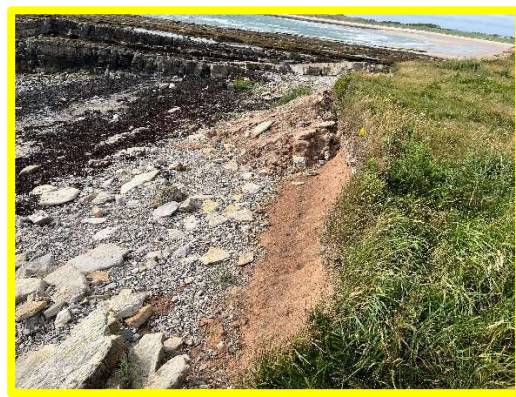
Slumping of cliff material adjacent to Long Sea Outfall (LSO) (1701C22)
