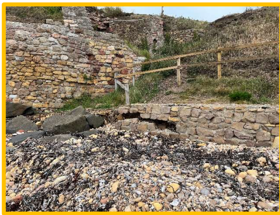
Damage to retaining wall adjacent lime kiln. (1701C45)
