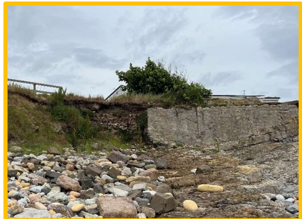
Outflanking of wall to north of gabions (1701C38)
