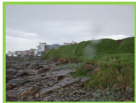
1701/C54 – slight erosion
