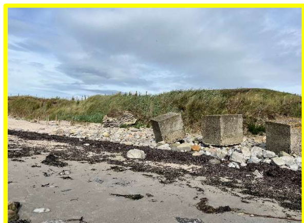
limited erosion to golf course 1701C23
