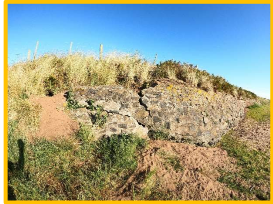
1401C27 – Localised section to the north of mortared revetment failed. Extensive cracking and washout of material.
