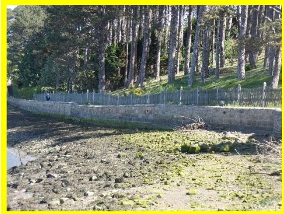
2801/C10 Local undercutting of concrete toe to repaired section
