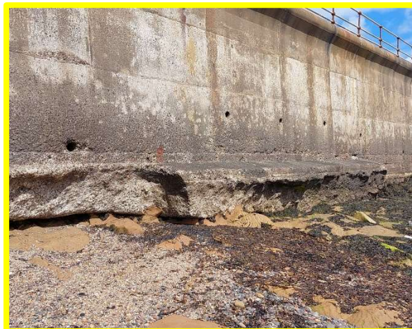
Church Point seawall in fair overall condition with localised undermining of toe protection (/3601C12)
