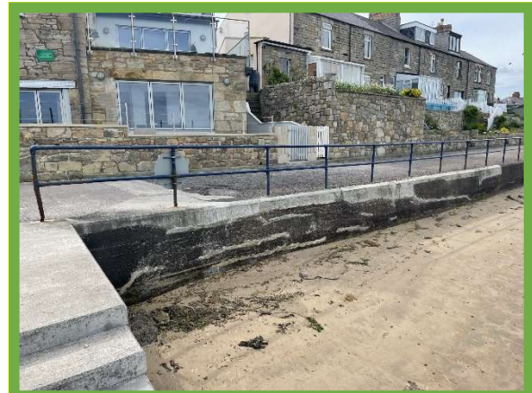
Seawall at Little Shore Wave Basin repaired to good condition in 2020 (/3001C10)
