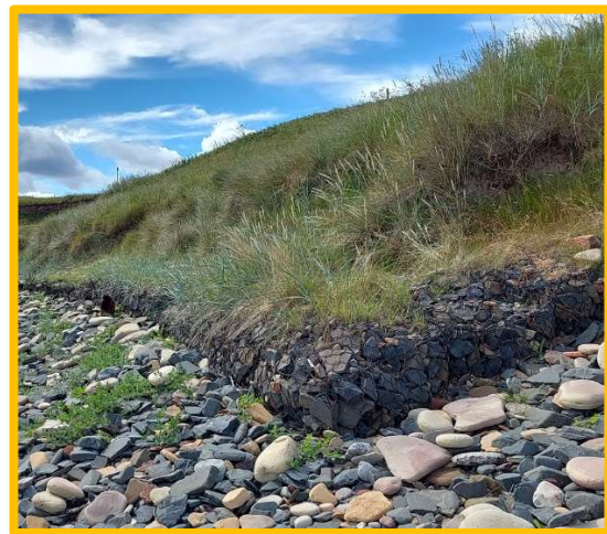
Gabions failing and slumping cliff (/3201C22)
