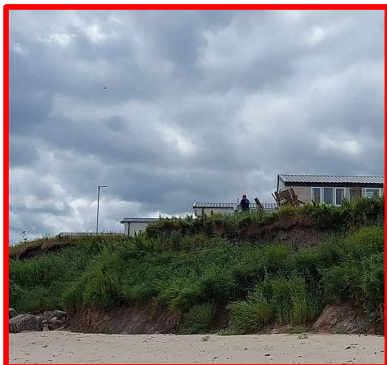
Active slumping at northern section fronting caravan park (/3501C05)
