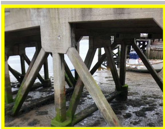
901c06 - spalling to RNLI structure.
