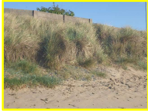
Very narrow dunes with gabions at toe becoming exposed (/4201C11)
