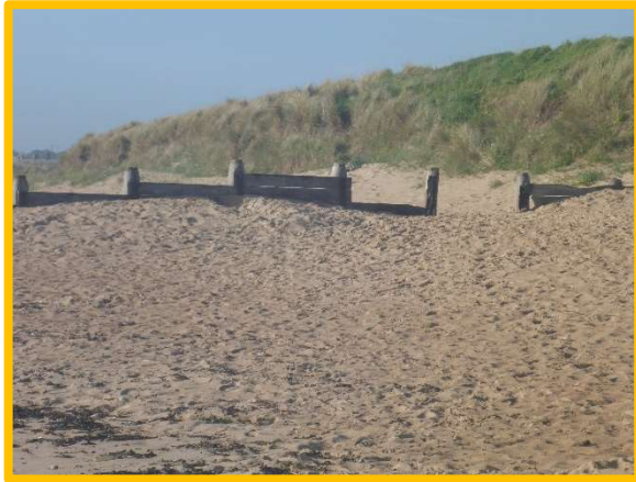
Central groyne (/4301C01) – poor condition
