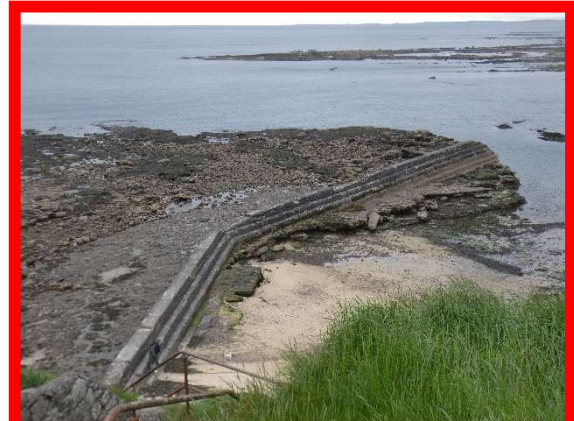
Damaged section on breakwater crest (/0701C04) 2022. Further damage and undermining.
