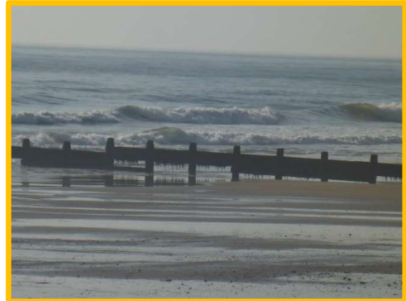
Central groyne (/4301C01) – poor condition
