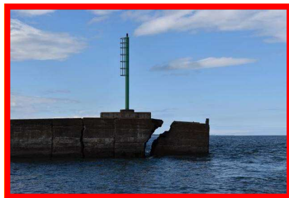
Seaward end of North Pier in very poor condition (/3001C02)
