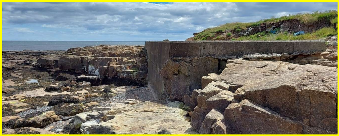
Seawall with undermining and outflanking (/3501C08)
