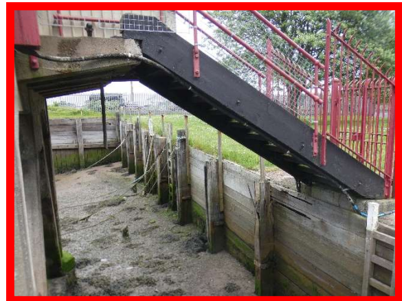
901c06 – loss of integrity of timber retaining wall.
