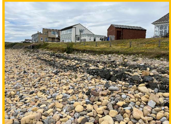
Erosion bypassing the gabion baskets (1701C40)
