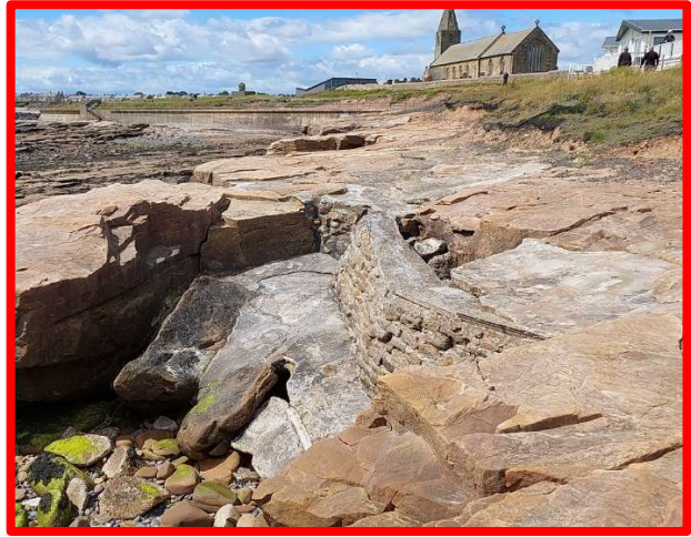
Voiding at crest of small wall in 2020 (/3601C01)
