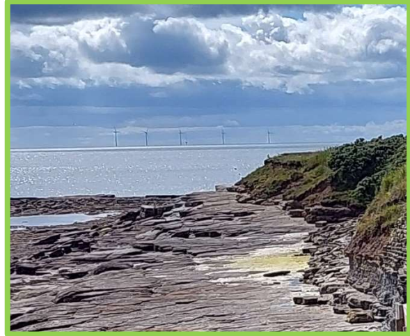
Slumping soft cliffs above rock ledge around Snab Point (/3301C01)
