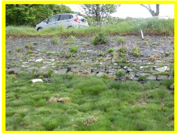
1501/C04 – very local undermining due to back creek development.
