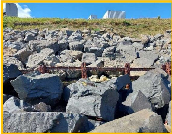
Steel framework separating old and new rock armour – no need for repairs as it has no function due to new rock armour below (/4001C02)
