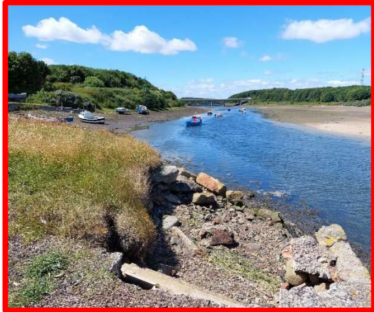
Wansbeck Boat Club retaining wall leeward erosion – local defect (/3801C02)
