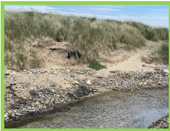
View from landward to seaward of ‘daylighted’ open channel section of outfall from Hauxley Nature Reserve, exposed geotextile in black (/3201C09)
