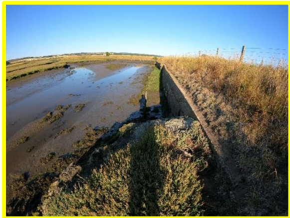
1401C15 – Concrete wall in fair condition. Timber toe erosion protection in poor condition.
