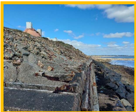
Industrial waste that looks unstable and could collapse over the structure (/4001C03)
