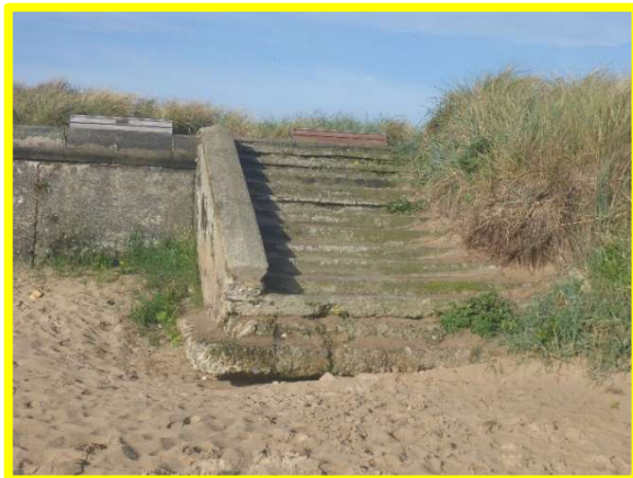
Abrasion and undermining of access steps (northern end of sea wall) to seawall (/4201C06)
