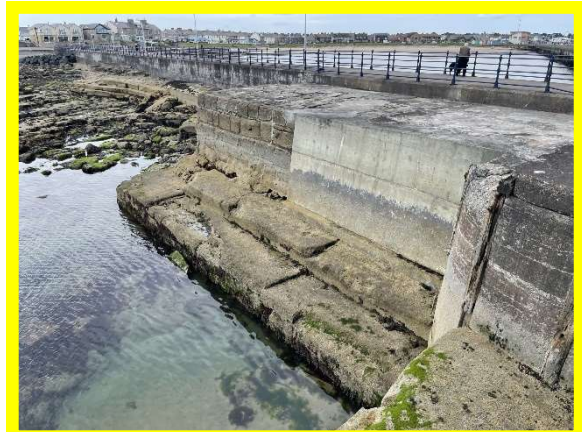
Repairs at junction of South Pier and South Jetty (seaward face) made in 2018 (/3101C01)
