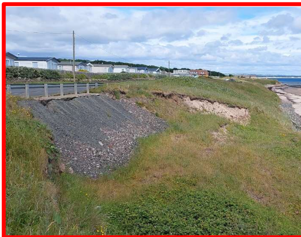
Failed section of cliff adjacent to coast road (/3201C22)
