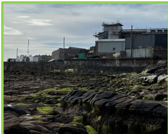
Storage yard wall in good condition (1701C05) Significant cracking to parking area wall (1701C06)
