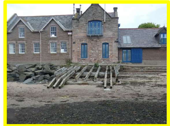
Obsolete timber slipway (/0801C05) 2022
