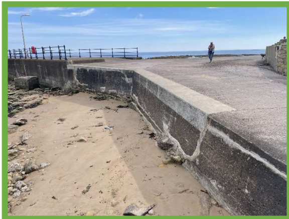
Repairs return sea wall along Bay View to good overall condition in 2020 (/3001C10)
