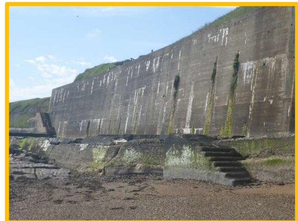
Abraded toe apron of sea wall (/4401C17)
