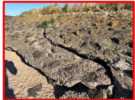
1401C29 – Failed section of the grouted stone revetment.
