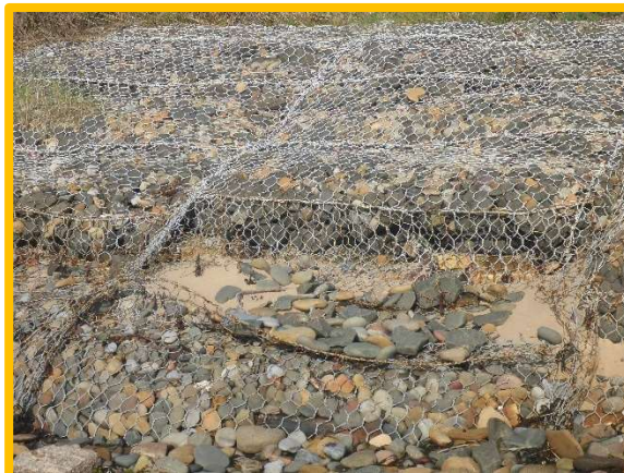
One example of several failed gabions (/4201C03)
