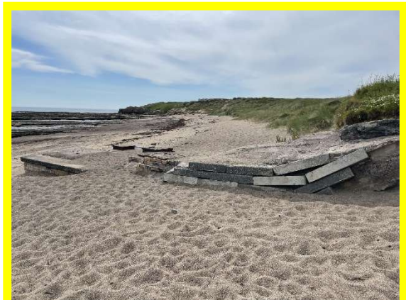
Dilapidated but largely buried outfall (/3101C09)
