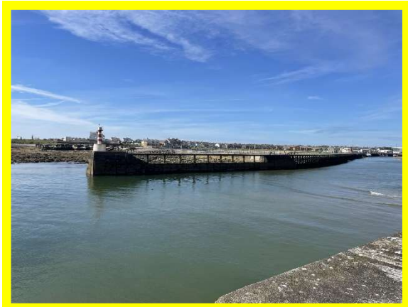
South Pier in fair condition, possibly some voiding at base. (/3101C01)
