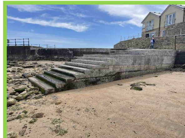
New access steps to Little Shore Wave Basin in good condition in 2020 (/3001C10)
