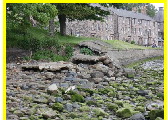
Western end failure of wall (/0801C07)
