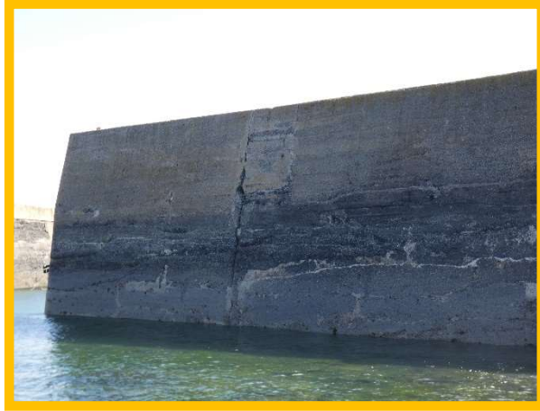
2201C03 Crack in north pier. No change
