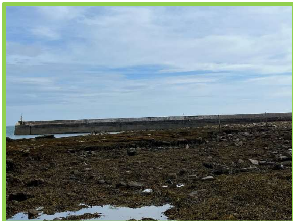
Damage to the cope stones noted – Inspection from afar only (1701C21)
