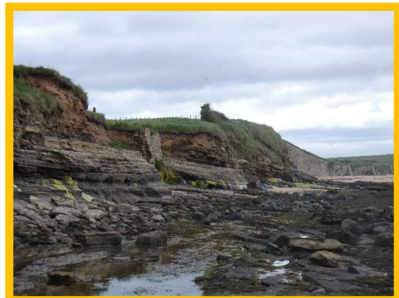
2501/C01 masonry wall in poor condition being outflanked.
