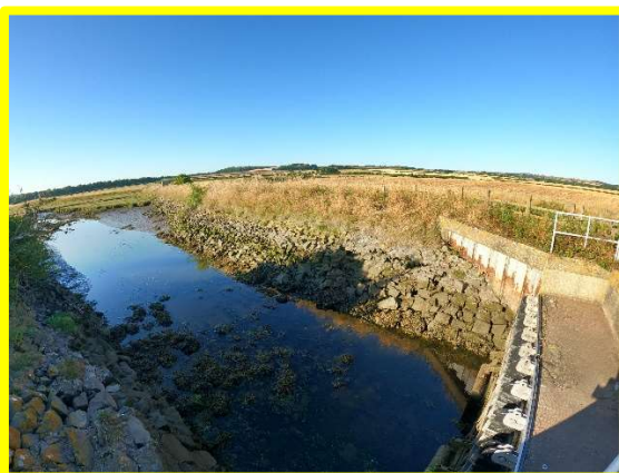
1401C17 – Uneven rock revetment profile
