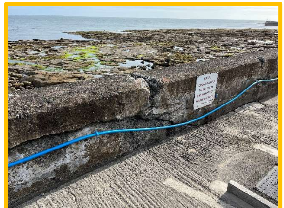
Significant crack through parapet wall (not worsened since 2020) 1701C06
