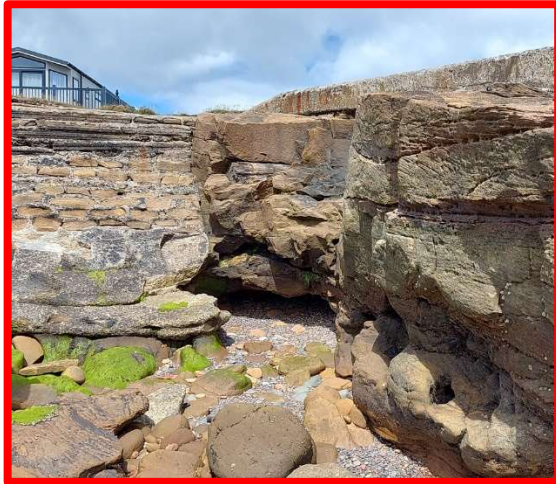
Severe undermining of masonry walls and rock ledge (/3601C01)
