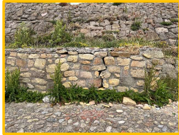
Significant cracking to the stone terraced structure (1701C45)
