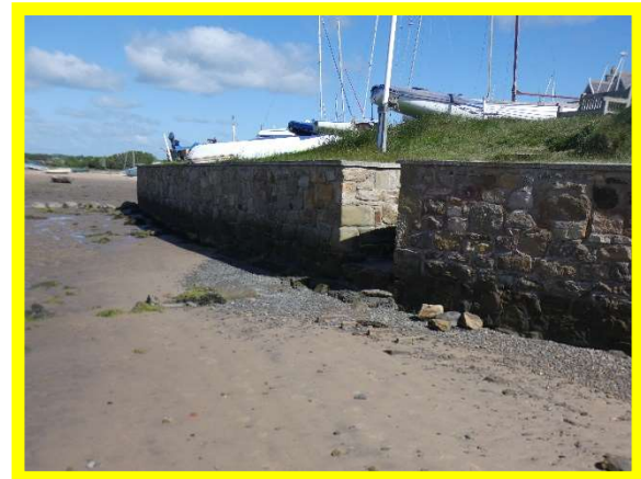
2801/C03. Masonry wall at Boat Club with slight undercutting. Little change.
