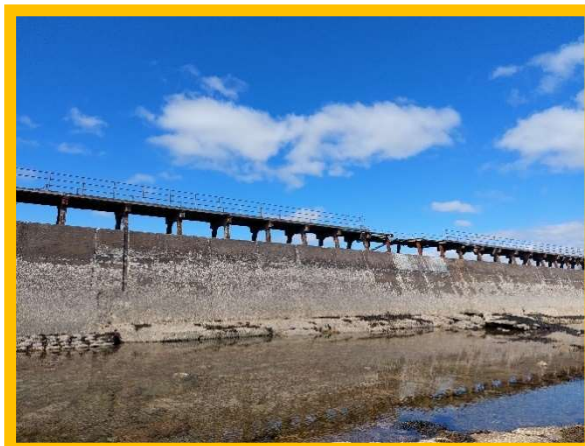
Seawall in fair condition – missing sections of trestle deck (/4001C05)
