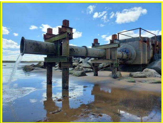
Power Plant water outfall through the rock revetment (/3401C08)
