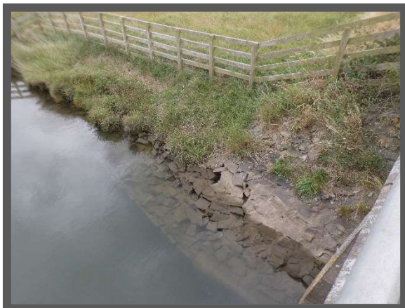
1401/C01 – 2020 undermining of edge protection.
