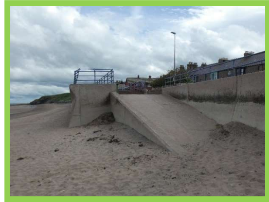
1001 c03 – 2022 slight reduction in beach level
