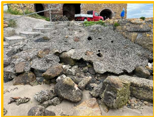
Undermining and partial collapse of grouted stone revetment adjacent access steps. (/1701C53)
