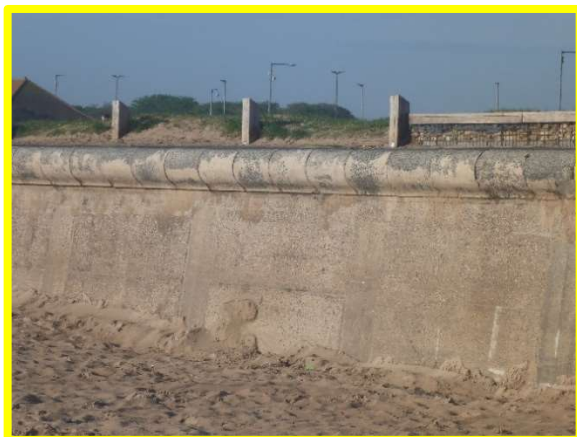
Sea wall fronting regenerated Blyth seafront – northern end of Blyth promenade (/4201C07)
