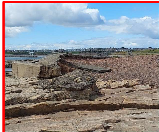
Second length of seawall with undermining and outflanking (/3501C10)
