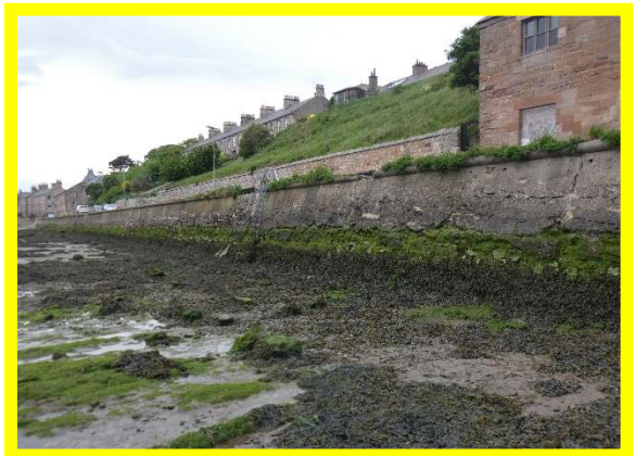
Deterioration of the coping (/0801C07)
