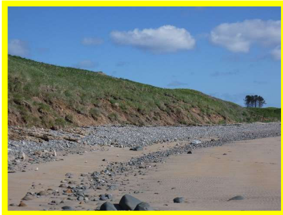
2701/C02 some slope failure continuing since 2018
