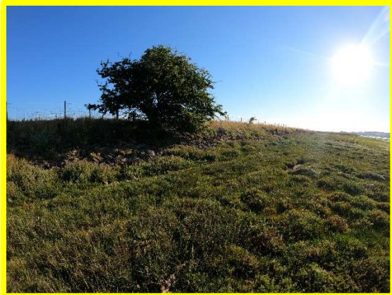
1401C27 – Mature vegetation growth through revetment.
