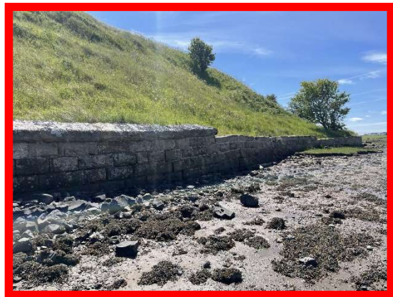
Movement along section of wall at Church Hill (/2801C13)
