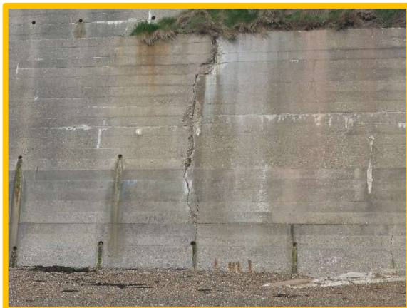
One of three notable vertical cracks in the sea wall (/4401C17)
