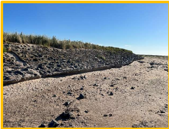
1401C29 – Undermining of revetment as a result of lowering beach levels.
