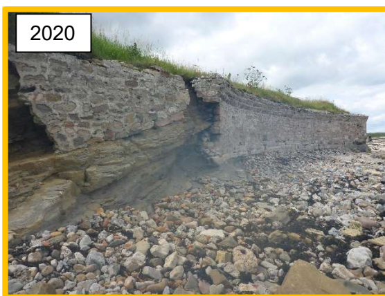
Masonry blockwork wall in poor condition. (1701C25)
