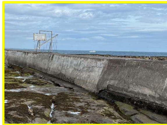
Horizontal cracking to seaward face (1701C20)
