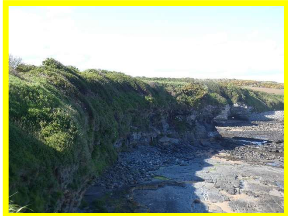
2401/C01 slow undercutting of cliff
