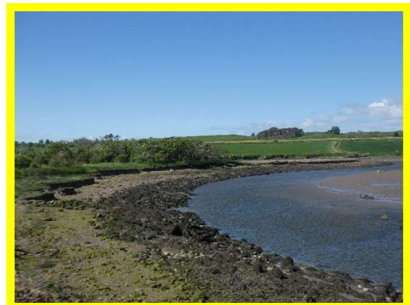
2801/C09 increased erosion 2022
