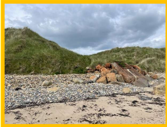
Rust-stained outfall within generally stable dunes (/3101C12)
