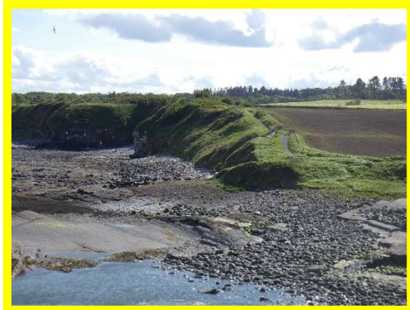
2401/C01 slow undercutting of cliff
