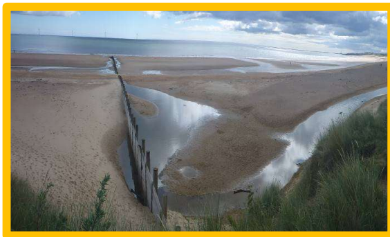
Meggie's Burn channel undermining southern groyne in 2020 (/4301C01)
