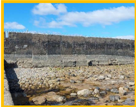
Sea wall that has experienced moderate amount of erosion – needs to be monitored carefully or repaired (/4001C04)
