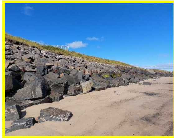
New rock armour placed at toe to create a stable slope, protecting the damaged steel (/4001C02)
