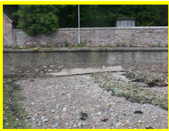
Eastern end undermining (/0801C07)
