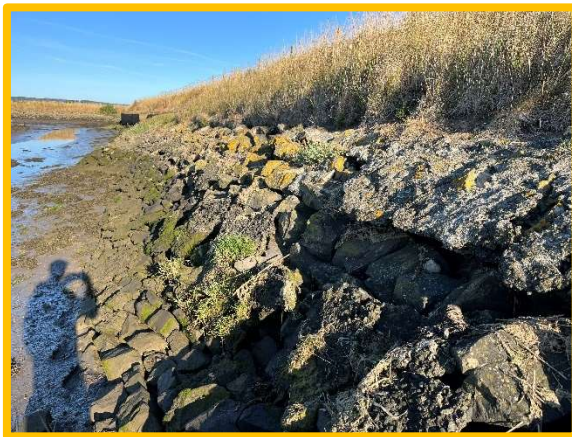
1401C14 – Grouted stone revetment in poor condition.
