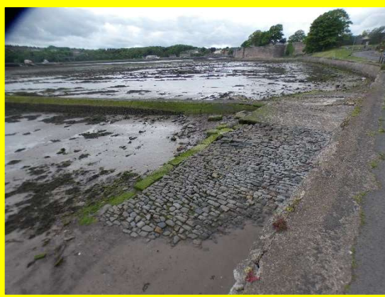
Local failed section of slipway over foreshore outfall (/0801C07)
