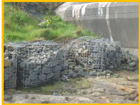
Break-up of gabion baskets (/4401C19)
