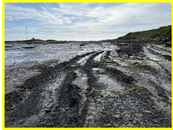
Heavily rutted foreshore fronting rubble (1701C19)
