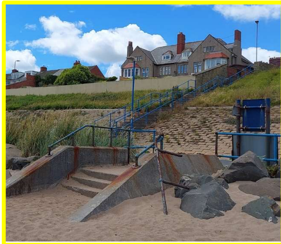
Healthy beach levels fronting rock revetment. Corroded handrailing and posts (/3601C08)
