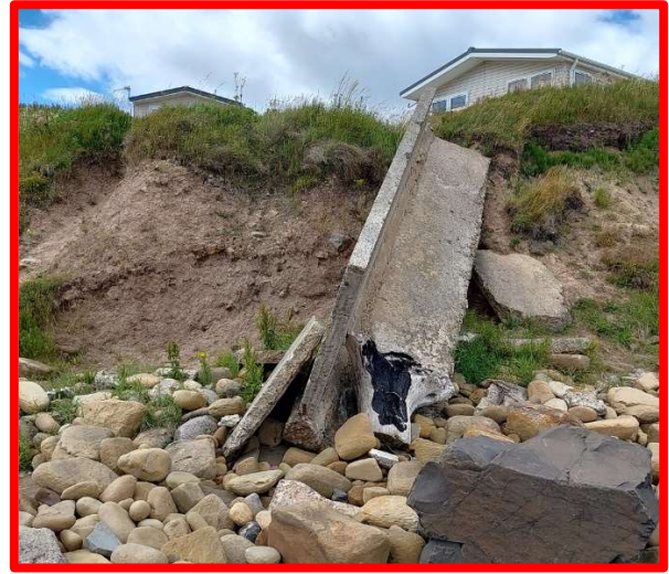
Erosion recommences to immediate south of rock berms (/3701C03)
