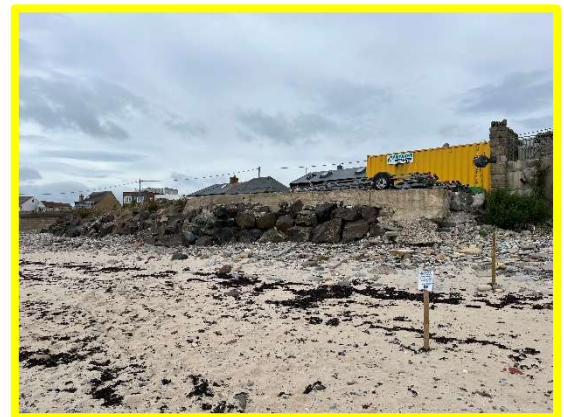
Concrete cast onto the crest of the revetment to provide flat storage area ( /1701/C32)
