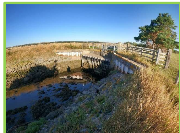
1401C18 – Good condition sluice at Ross Low channel. Corrosion on adjacent steel sheet piles.
