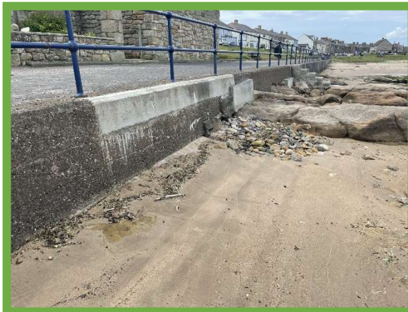
Repairs return sea wall along Bay View to good overall condition in 2020 (/3001C10)
