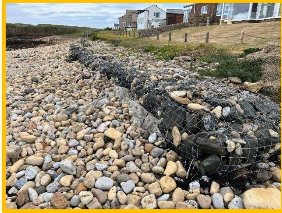
Damage to gabion basket wall at (Lady's Hole) gabion wall – partially submerged to high sediment levels. (1701C40)
