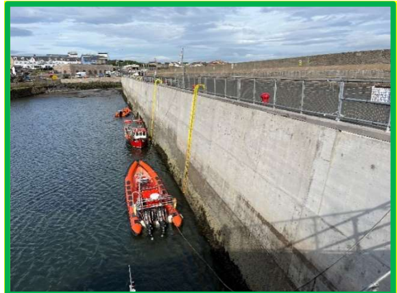
Concrete encasement and cope repair to inner face of north breakwater. 1701C09
