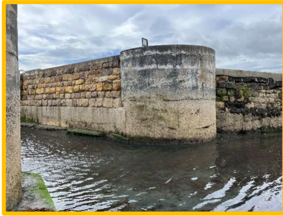
Undermining of Beadnell Harbour wall (inner face of southern wall) (/1701C51)
