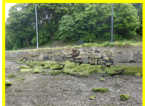
901c05/06 further cracking and loss of pointing 2022.
